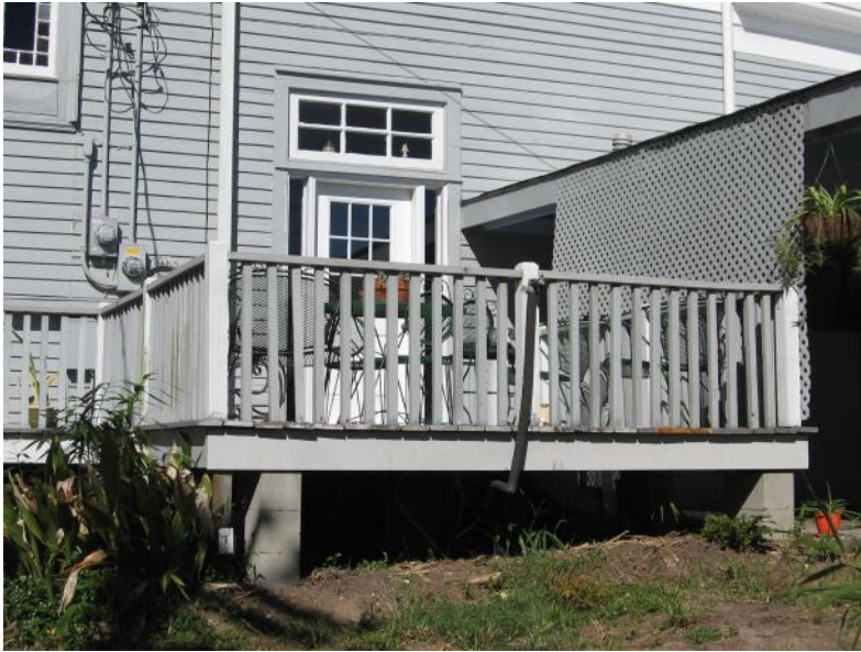
The deck at the rear of 132 S. Main Street is an appropriate example of a compatible deck addition (above). Decks should be added at rear elevations where they are not readily visible (below).
