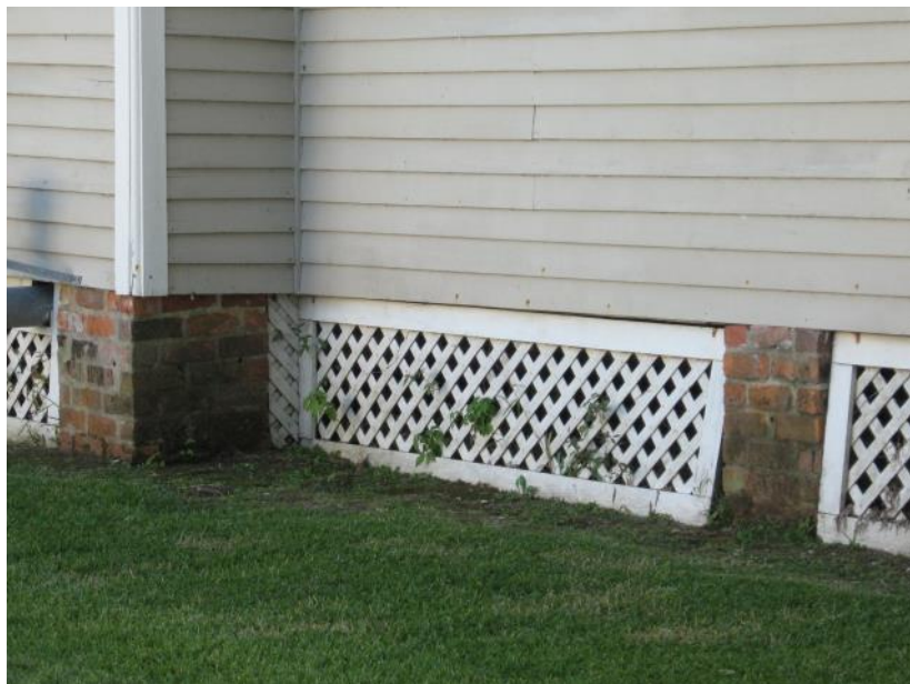
The use of frame lattice panels between brick piers is appropriate for most dwellings in Abbeville. They assist in ventilation and help secure the area beneath the house (207 S. Washington Street).
