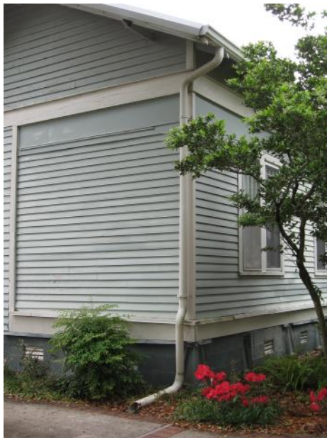
The gutter and downspout at 208 S. Washington Street directs water away from the foundation of the dwelling.
