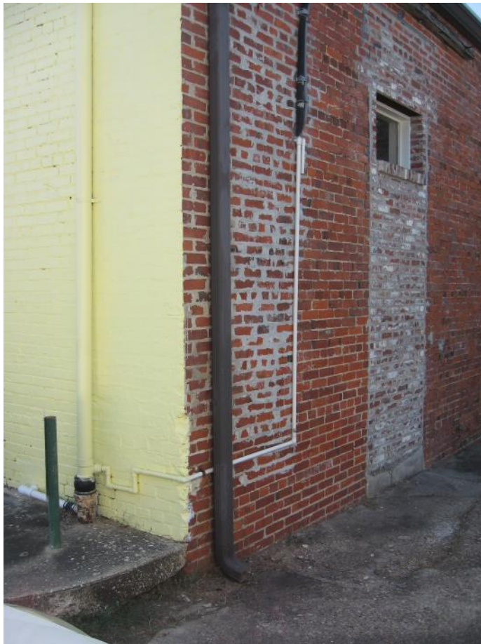
Gutters should be placed on rear elevations and be of a color to blend with the building such as at the rear of 214 S. State Street.
